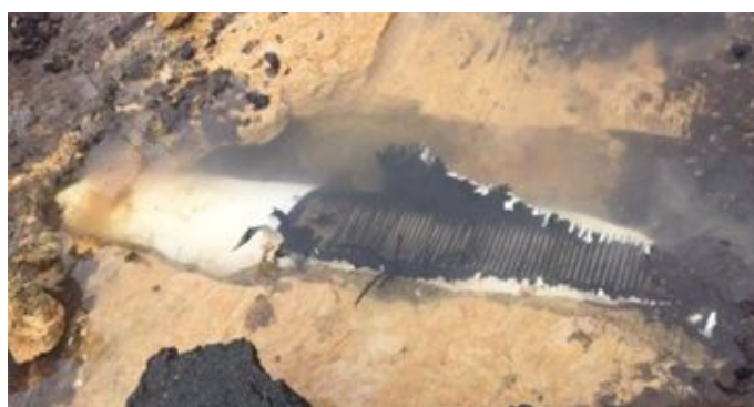
Damaged Glenvar No.1 Watermain
